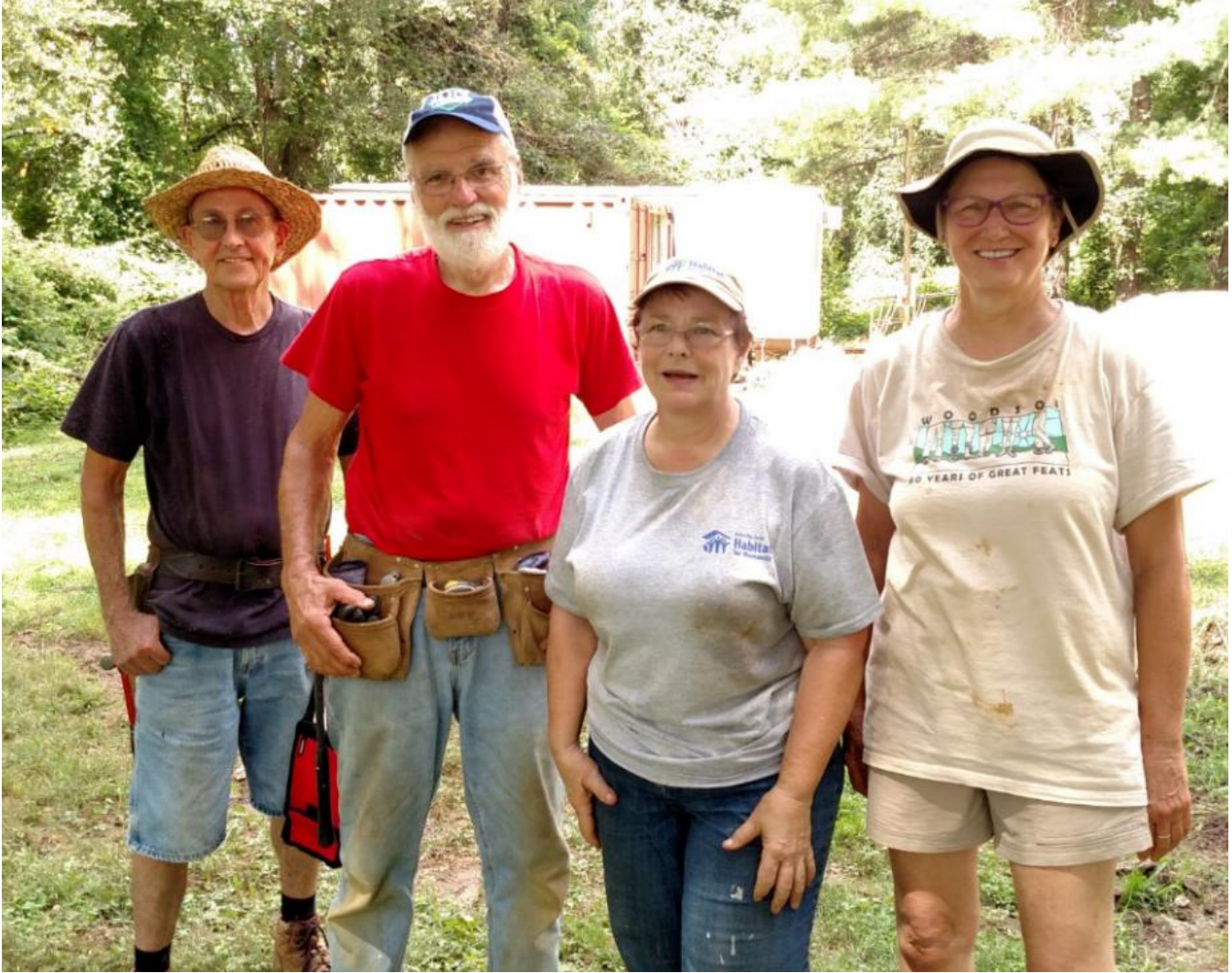
WWPC volunteers helping get construction of Presbyterian/Methodist House # 25 underway on Aug. 11 included Bill Heck (left), Toby Ives, Georgena Millar and Sally Broughton.
