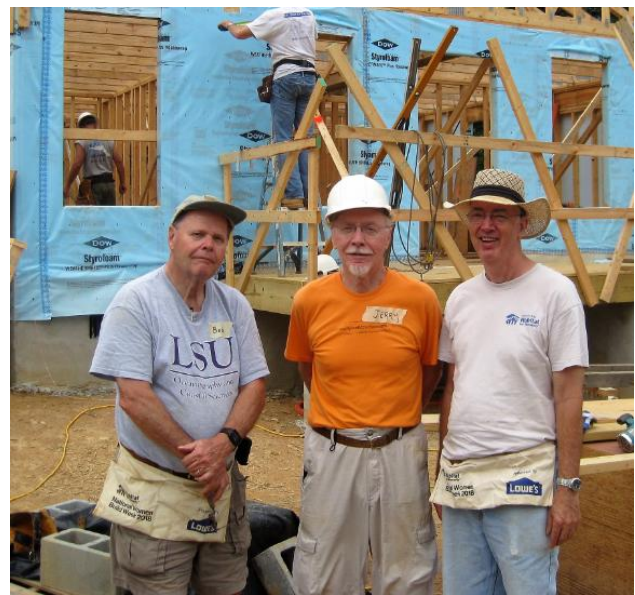
Bob Gambrell, Jerry Vaneman and Larry Griswold worked on the house on Aug. 22 doing interior Framing and helping prepare for installation of the roof.
