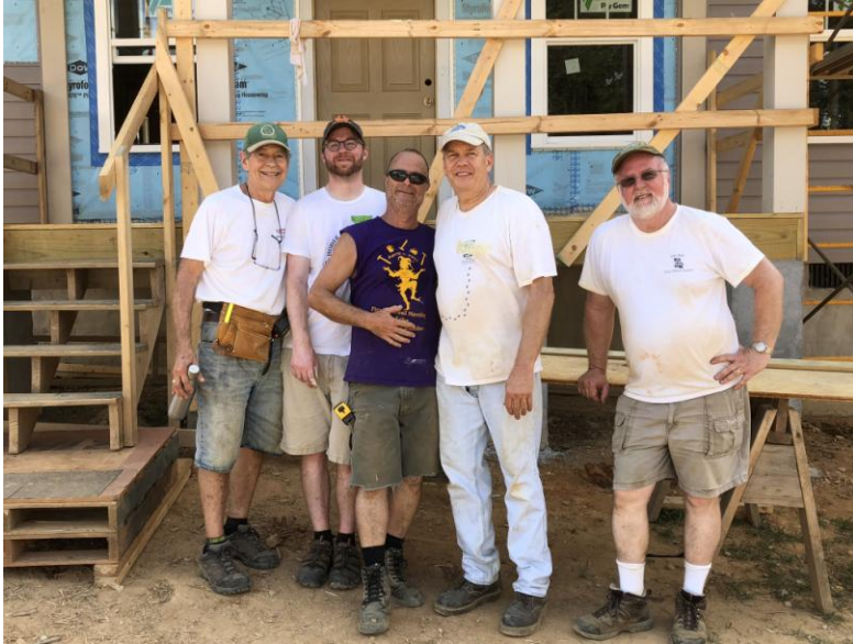
Ned Guardenier, Andrew Daugherty, Brent Roberts and Derron Daugherty worked with Habitat Construction Supervisor Craig Comeau (center) to cut, fit and install siding on the house.
