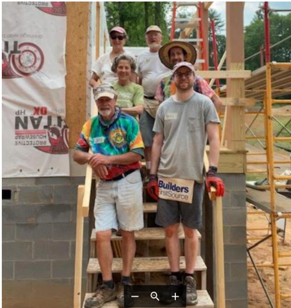
HELPING BUILD THE HOUSE OF FAITH on May 21 - front row, l. to r., Habitat core volunteer Jerry Ray, Andrew Daugherty; second row, Betsy Warren, Construction Supervisor John McDermott; back row, Sally Broughton, Don Collins.
