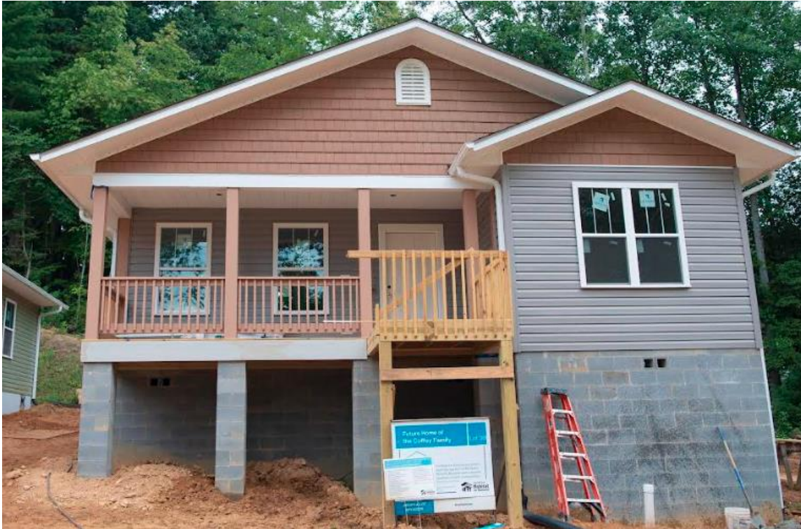
Construction of the Habitat for Humanity House of Faith began less than five months ago, and this photo was taken in August.
